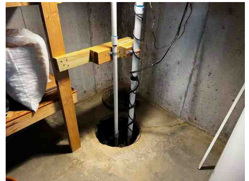
Basement Sump Pump
